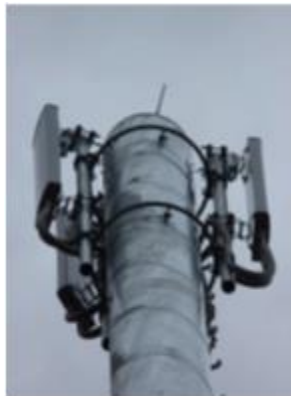
Fig. 4: Typical view of the top of a three sector cellular base station tower
